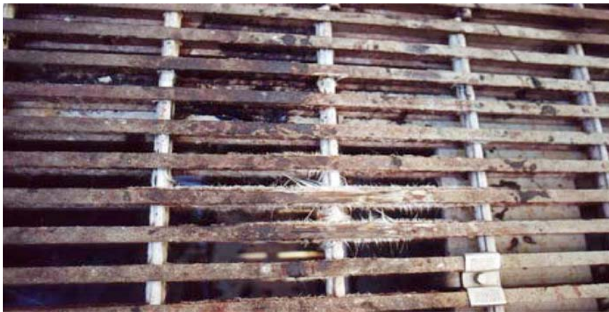
FIG. X1.11 Damage to FRP Gratings from Chemical Exposure
