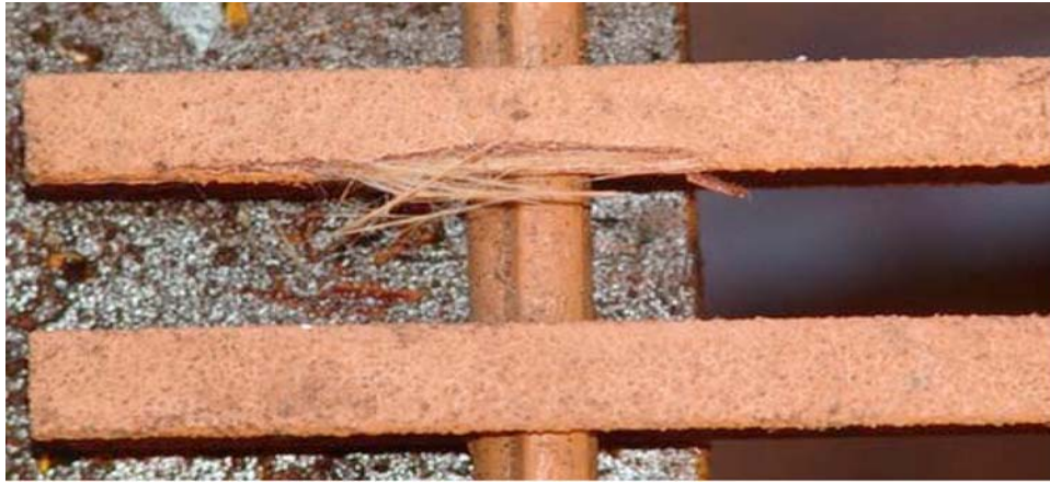
FIG. X2.5 Nonstructural Cosmetic Damage
