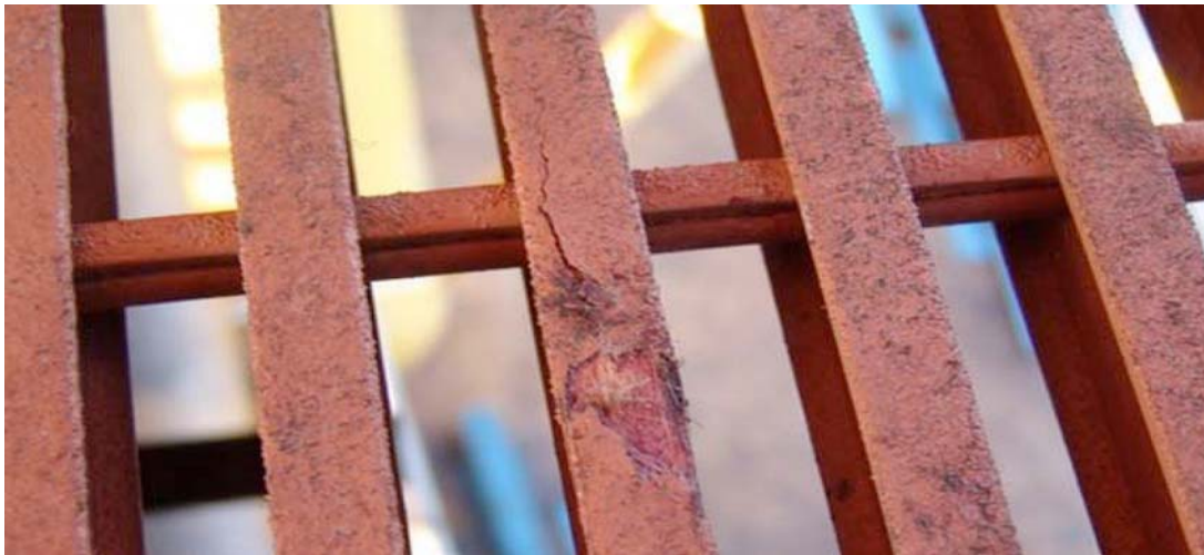
FIG. X2.6 Nonstructural Cosmetic Damage
