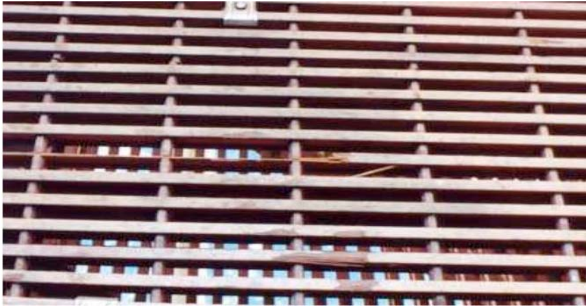
FIG. X1.10 Damage from Improperly Pulling Equipment over FRP Gratings
